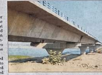
The work on a bridge over the Yamuna in Faridabad district was stopped due to the imposition of the model code of conduct.
